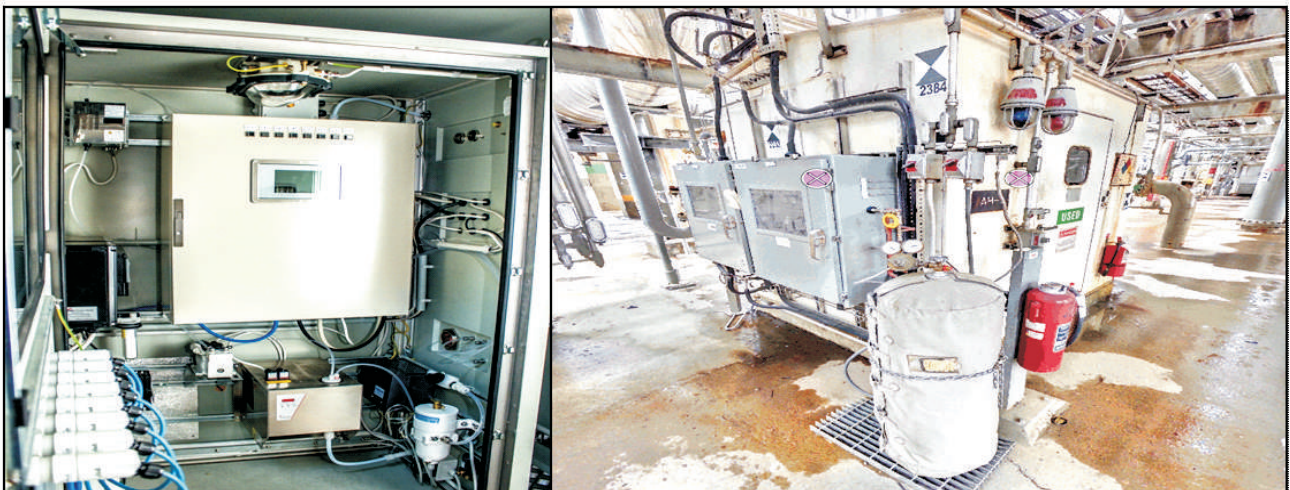
Figure 7. Sealed Cabinets or Enclosure
