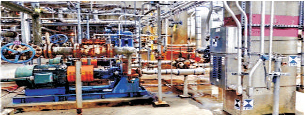
Figure 6. Purging Systems of Cabinet in Plant
