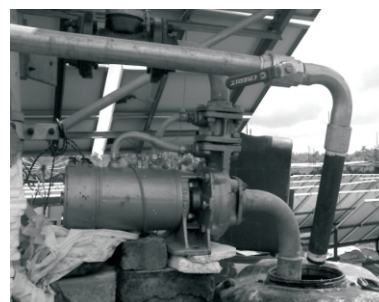
Figure 16. Photograph of the PMDC motor pump.
